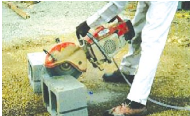
A worker cutting concrete block using a handheld saw that applies water to the blade. The water reduces the amount of silica-containing dust that gets in the air.
